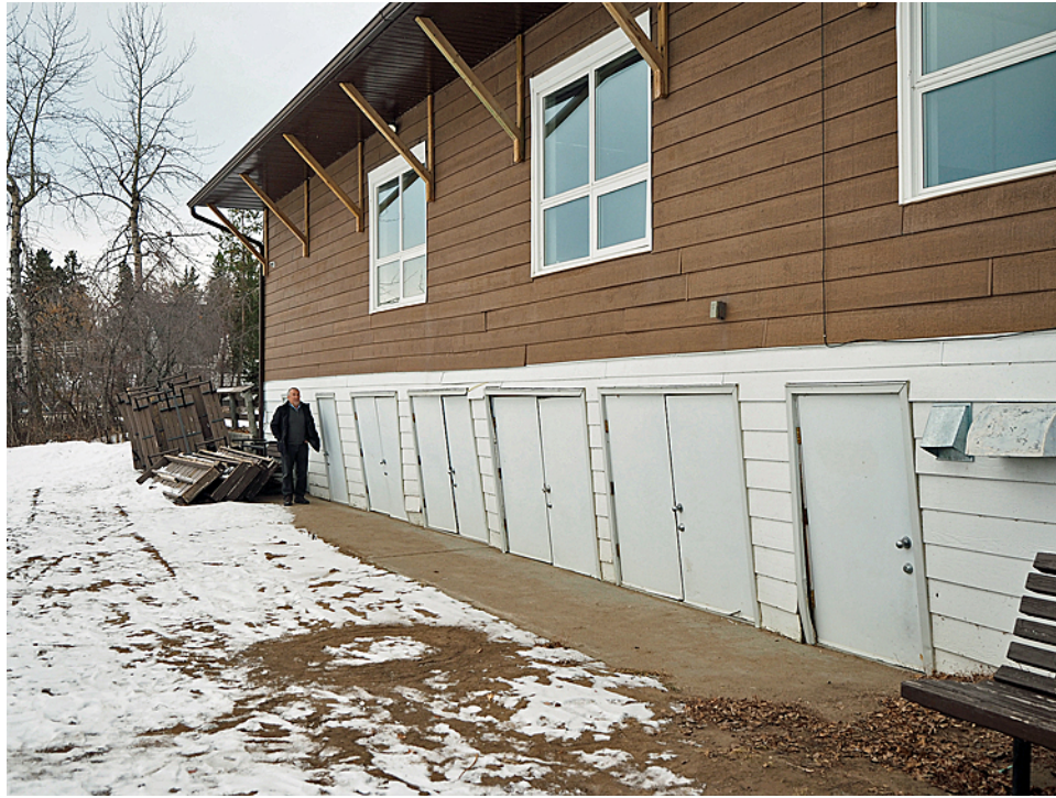
Although there was a ridge of debris in front of the pavilion, the ice shoved a concrete slab into the building, causing structural damage.
