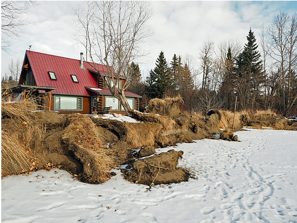
On the ground photograph of the damage in front of the red-roofed cottage in the previous UAV image
