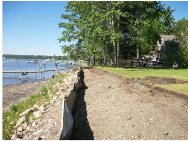
First step: removing the retaining wall and fire pit and installation of silt fence
